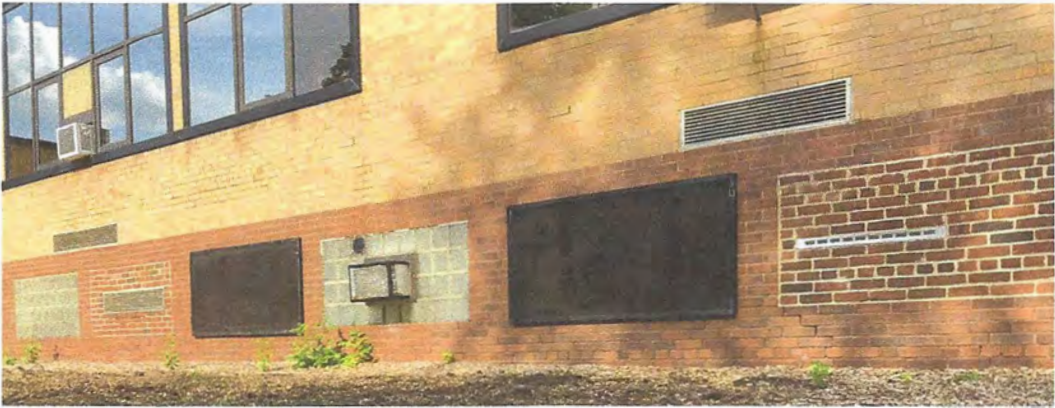
Above photo shows current state of basement windows with several instances of complete elimination.
