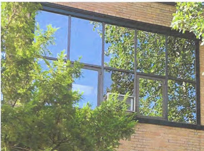
Present day windows. According to Northville Public Schools, the windows were replaced in 1990. The design was changed presumably due to problems with leakage. Similar changes were made on the western side of the building.
